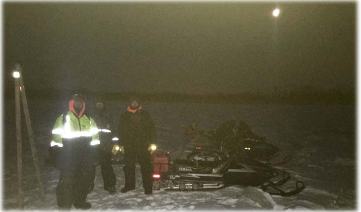
With barely 6 hours of daylight in mid-December some of the work gets done in the dark. Here the Kalskag trail crew is ending their day 18 miles from Home
