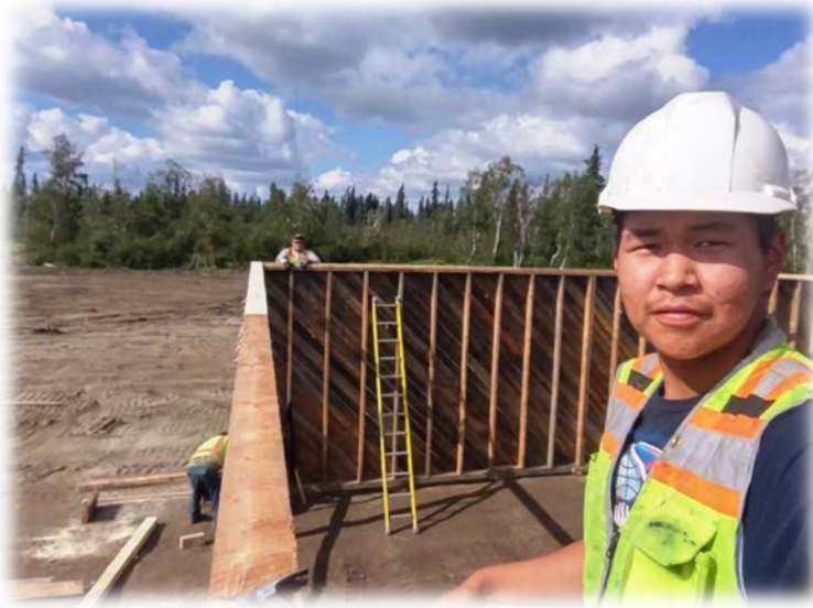
The Walls of One of the Sawmill Buildings Go Up on a Rare Day of Good Weather
