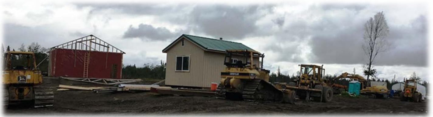
L-R: large storage building going up and the nearly completed office – just needs wiring
